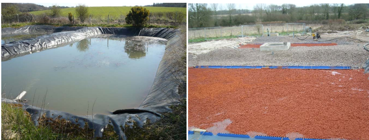
Fig 1: Tertiary settling pond at Wessex Water's Cranborne WTP prior to retrofitting (left); the same settling pond after installation of the technology (right).
