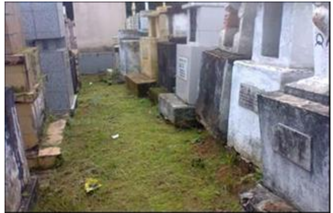
Fig 2: Structural conditions of the graves in Escada cemetery. Source: The authors.
