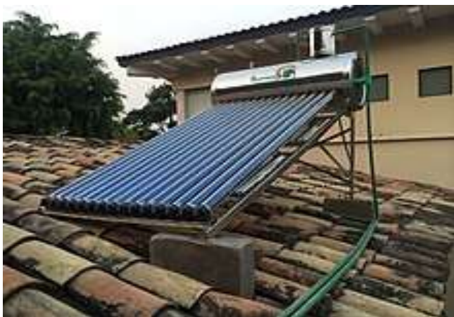
Plate 1: A Vacuum tube solar water heater on a roof
